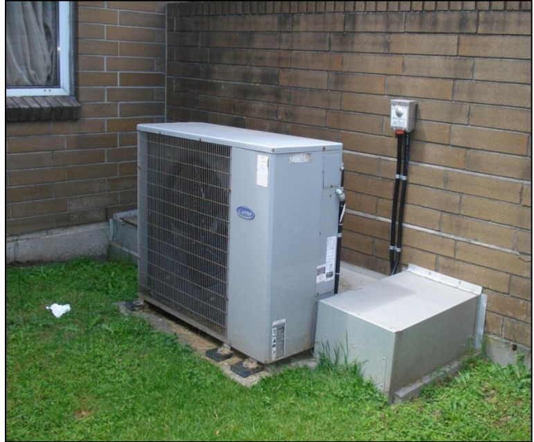
Air source heat pump installed in the back yard of a townhouse unit at Culloden Court.
