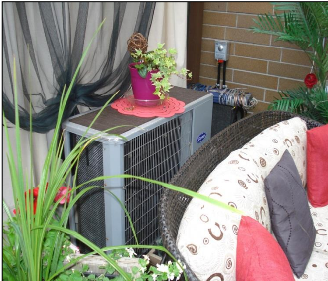
Example of an integrated air source heat pump with the back yard furniture of one of the townhouse units at Culloden Court.
