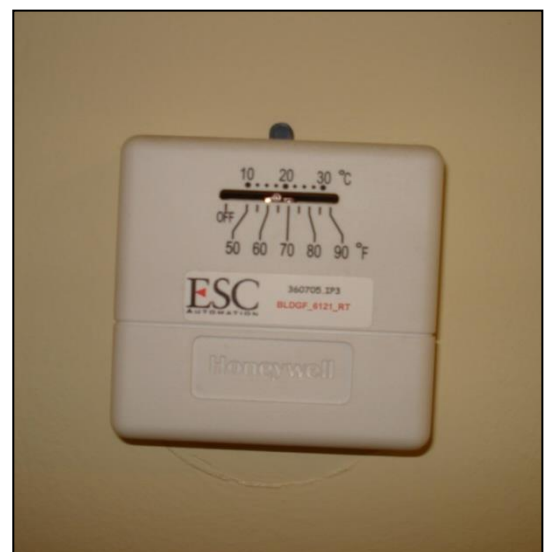
Typical thermostat installed at Culloden Court.
