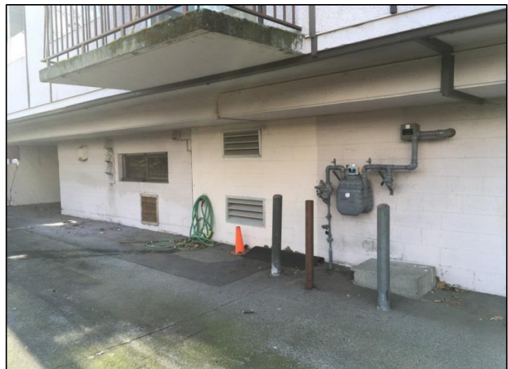
Outside area where the CO2 heat pumps are planned to be placed.
