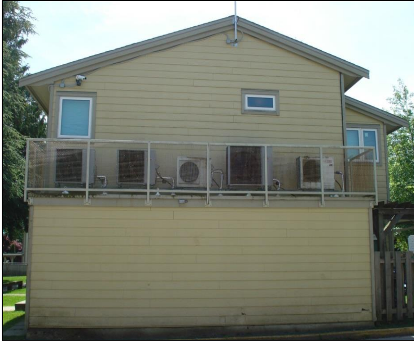
Back of Greenbrook townhouse row showing three new Arcoaire HPs (bigger units in grey) and two old HiSEER HPs (smaller units in white).
