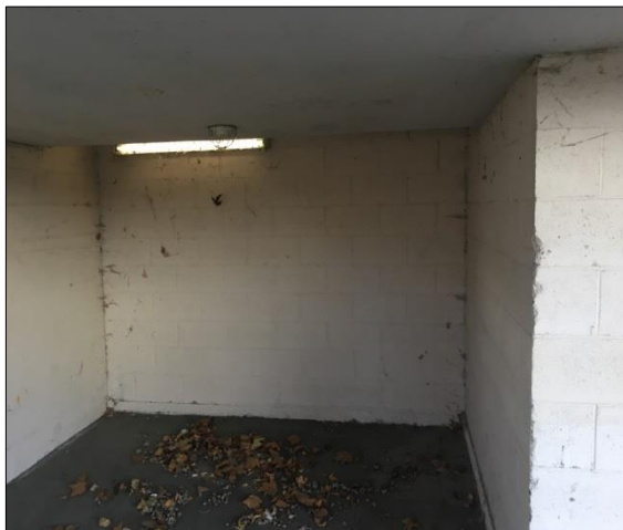
Covered parking area which would be used to house the storage tanks.
