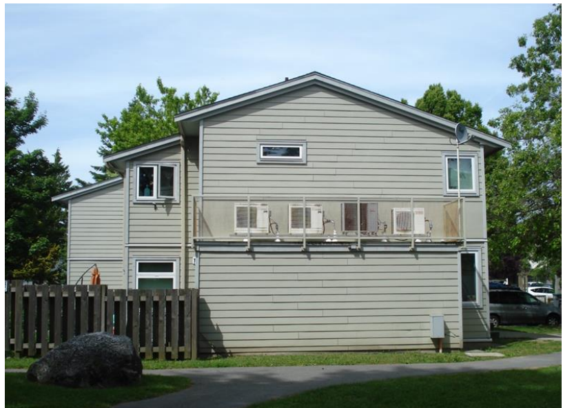
Back of Greenbrook townhouse row showing the elevated location of four ASHPs set up next to each other.
