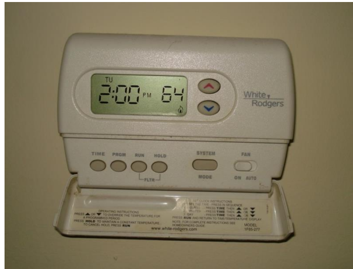
Typical thermostat installed at Greenbrook.
