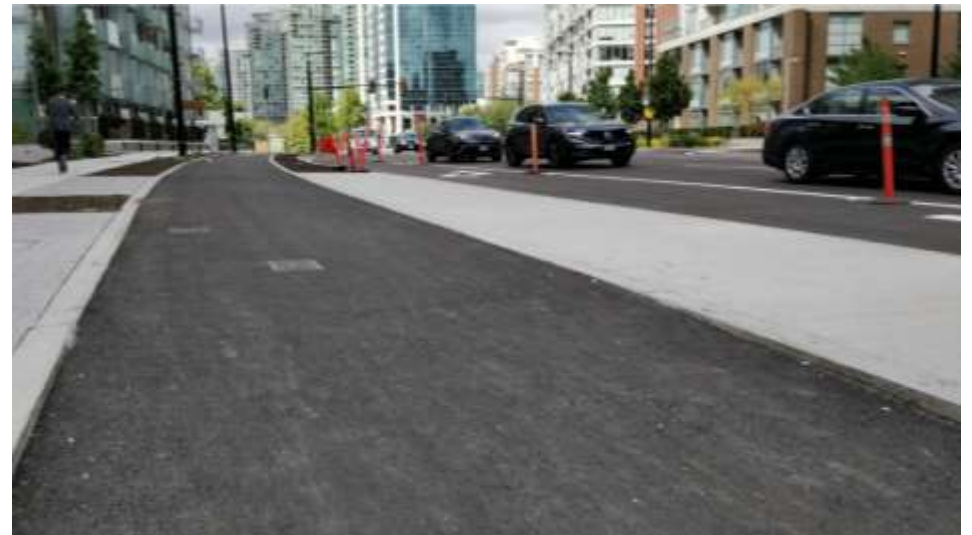
Post-construction looking north on Quebec St. The asphalt bicycle lane is covering
