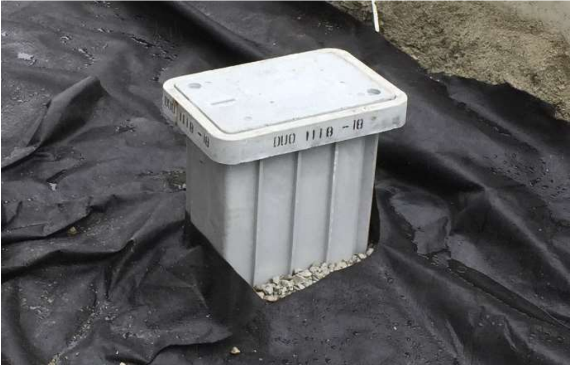
Figure 47: CoV standard valve box. Source: GI Branch
