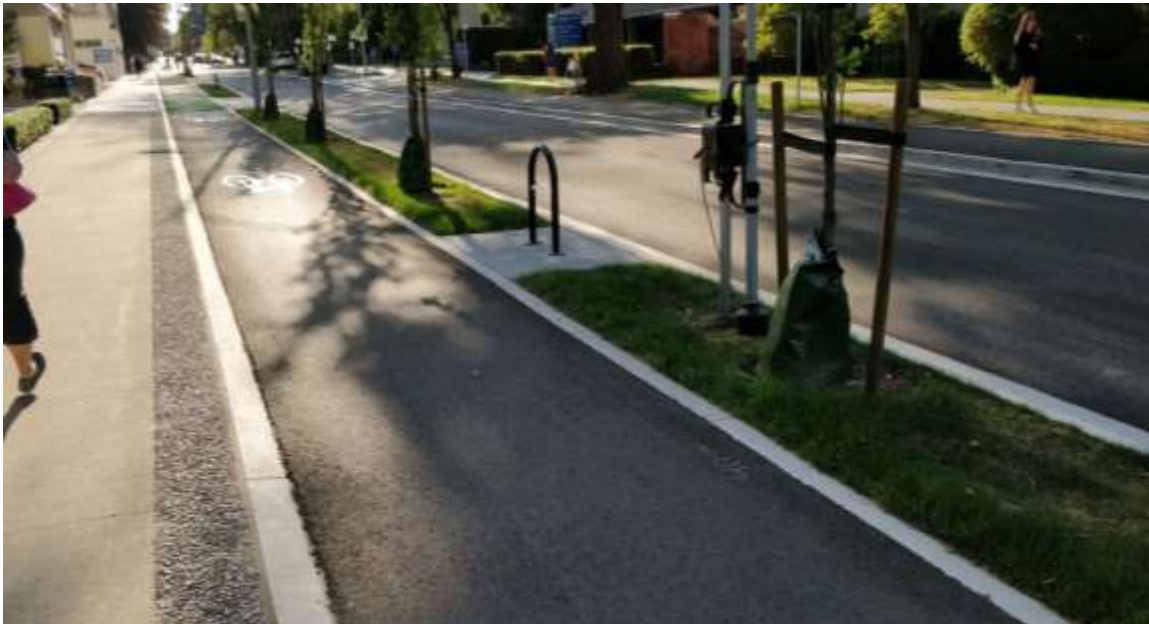
Structural Soil post-construction looking west. The asphalt bicycle lane is covering the structural soil
