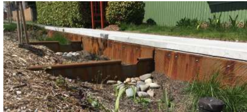
Figure 9: Soil cells used to support sidewalk and increase storage capacity in Ballard Neighborhood rain gardens in Seattle, WA.
