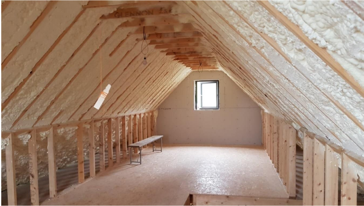
Figure 5. Sprayfoam insulation in an attic. Photo by U Value, 2017, via https://uvaluesprayfoam.ie/applications/attic-insulation/ .
