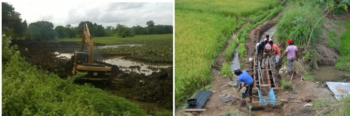
Fig 19. Restoration of the tanks in a cascade system according to the hydrology of the system in Kappirigama. Source: IUCN 2023 cited in Malaka (2023).
