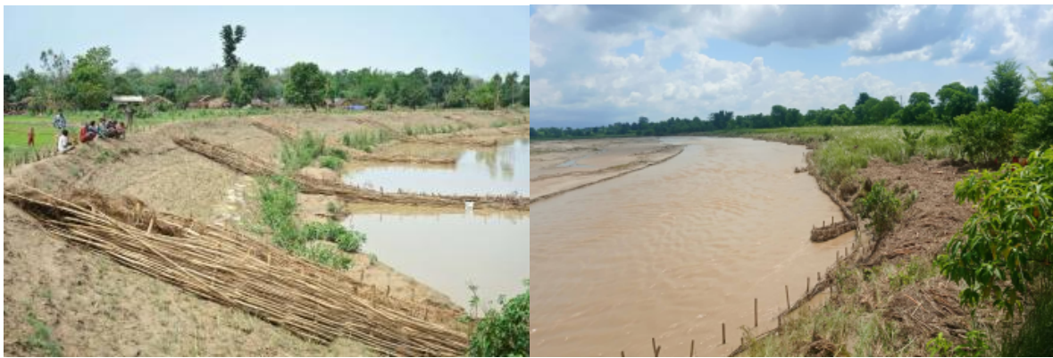
Fig 9. Community men and women-built bamboo spurs to hold the riverbank in place and planted kans grass to prevent flooding and erosion before the year's monsoon season. Source: Ojha (2021).
